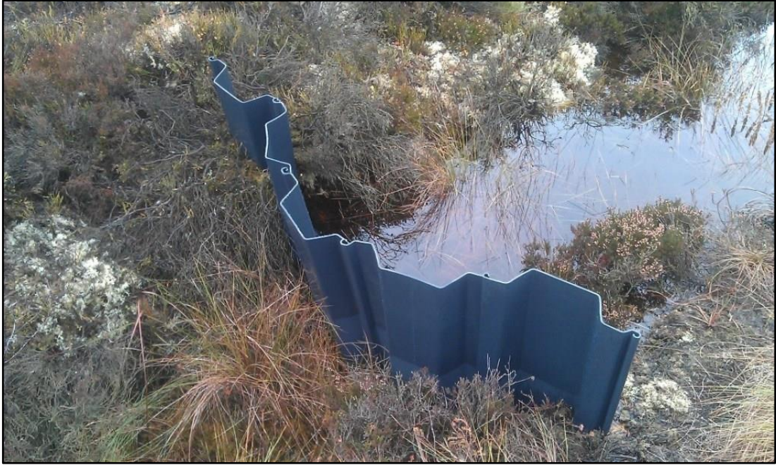
Plate 2.4 Example of plastic dams to be used for on-site drain blocking where peat dams are not suitable.
